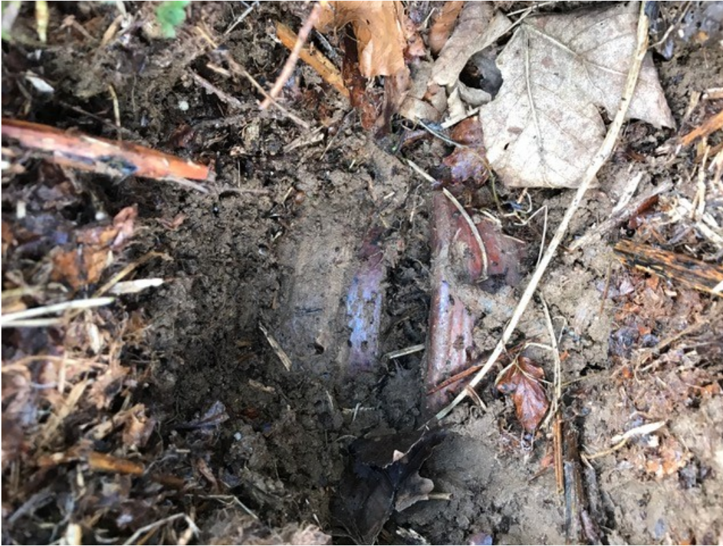
Structure 3. Open joint between two glazed pipes at base of small hole. (W Ward)
