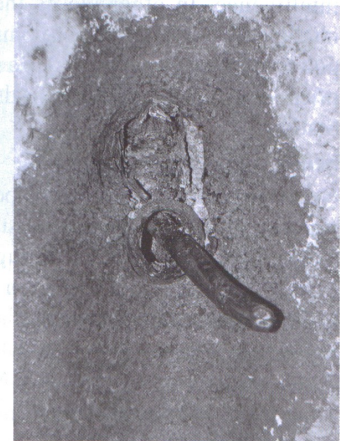
One of two two-cored 240 Volt mains power cables
