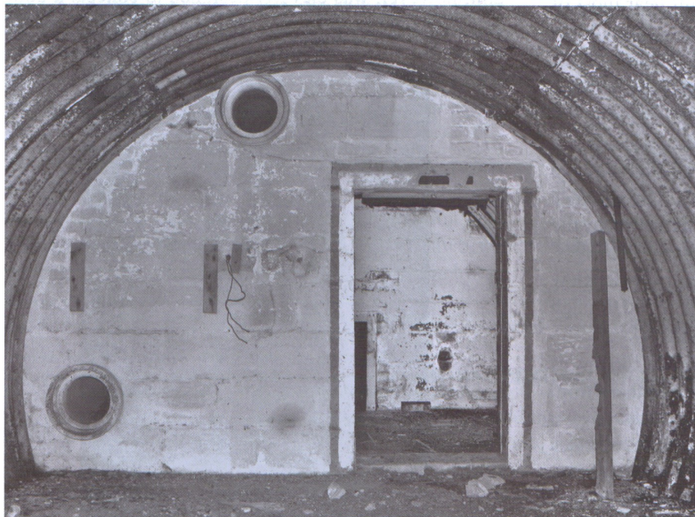
The operations room (view towards the generator room and emergency exit)
