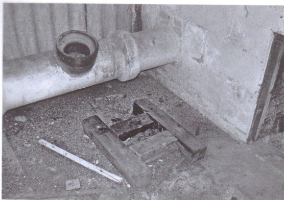
Wooden generator block
