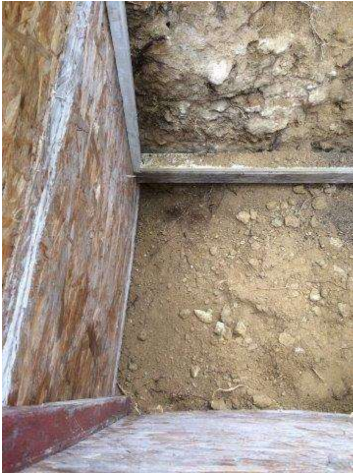
Pit where it was thought trap door was located. Three sides shuttered to prevent collapse. Third side limestone bedrock.
