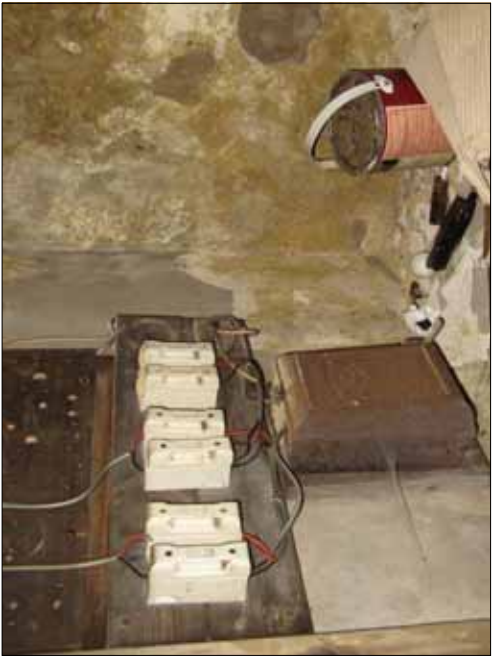
Plate 12: Possible circuit breakers in bunker
